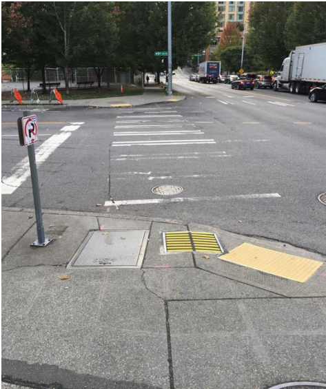
Figure 5. Photo of a corner crossing in Seattle showing a 2 ft x 2 ft square of raised bar TDI on the side of the DWS farthest from the center of the intersection for an apex curb ramp. The bars are oriented perpendicular to the direction of travel across each crosswalk (Bentzen et al., 2022). [Source: R. Wall Emerson]
