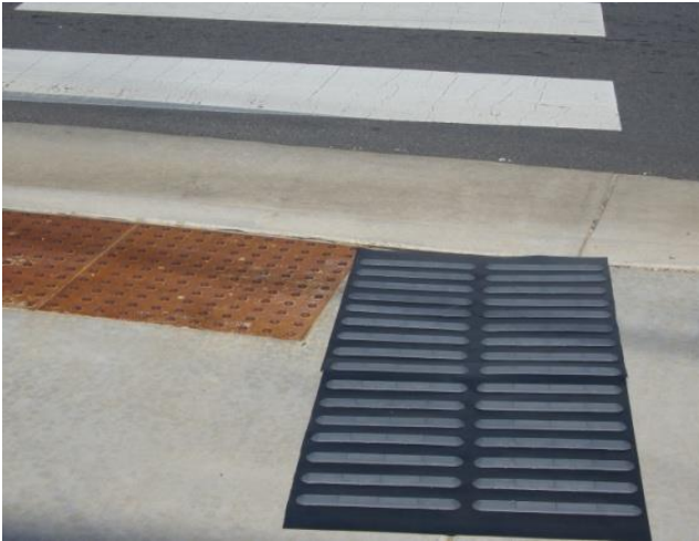
Figure 3. Photo of TDI with raised bars perpendicular to the direction of travel across the crosswalk, installed beside the detectable warning, found to enable efficient location of hard-to-find crossings and to significantly improve alignment for crossing by research participants who had little or no vision (Bentzen et al., 2017). [Source: B. Bentzen]
